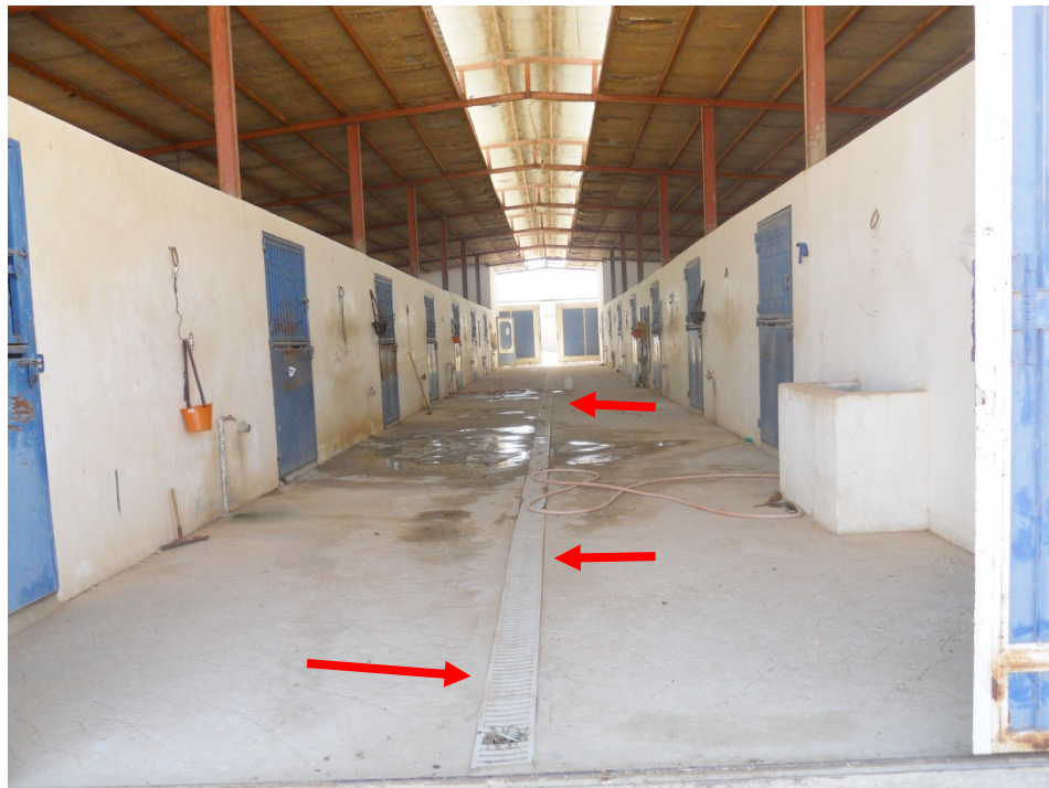
Center drain down length of stable where water accumulates
